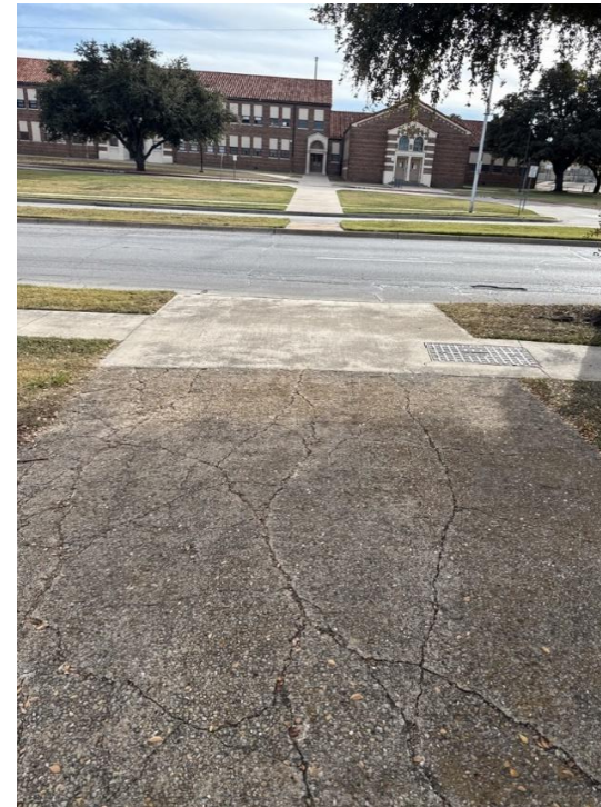
Midblock crossing of W Seminary Drive without curb ramps or markings
